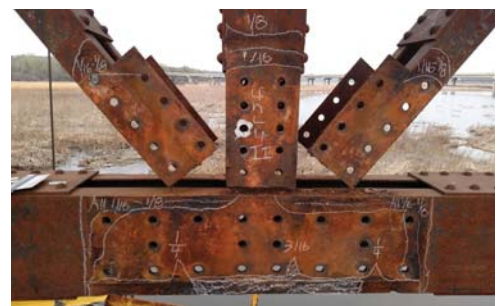
Deterioration Measurements on the Old Cedar Avenue Bridge (Refer to Challenge #3 on the following page.)
