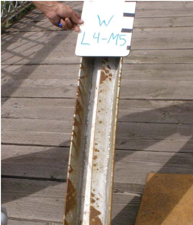
Vehicle Impact Damage on Bridge L5391 (Noted during SRF's 2009 investigation)
