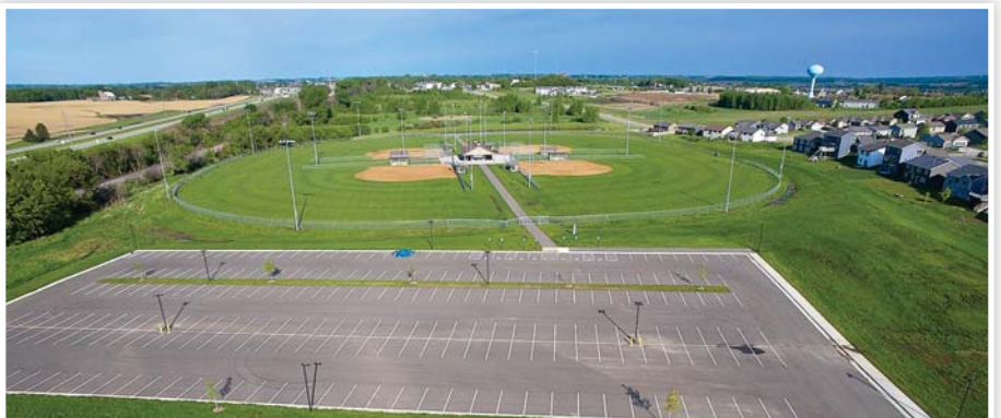
Construction of a 27-acre park that included four regulation-sized softball fields. The fields will host an array of teams from beginners to adult leagues.
