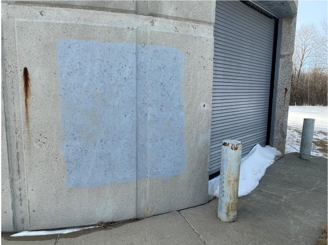
EXAMPLES OF RUST AND BLUE SQUARE SPOTS
