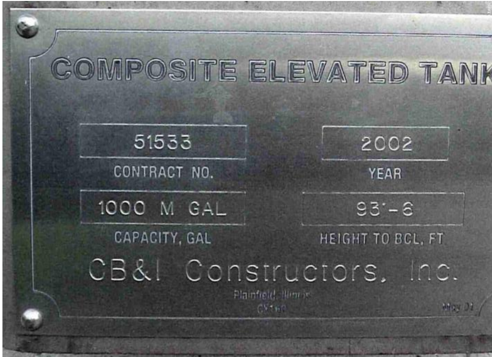
EXISTING WATER TOWER NAME PLATE
